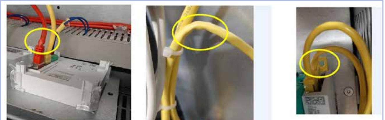
Fig. 13: Examples of poor RJ45 cabling.
